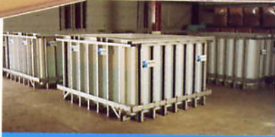
H 2 SO 4 pickling tanks.
