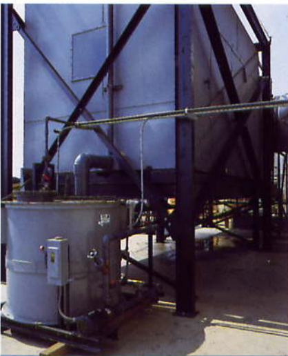
Tri-Mer tank used as scrubber recirculation vessel.
